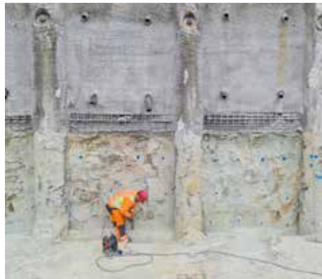
Layer by layer, the areas of quartzite rock between the bored piles are exposed.
